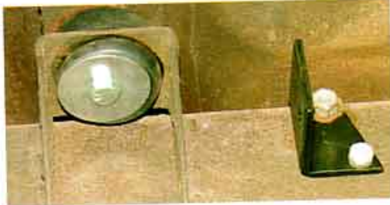
Photo #14: The body mounts that bolt to floor braces from the bottom use 2 1/2" bolts with 1 7/8" washers. Torque these bolts to 20 ft./lbs. as well.
