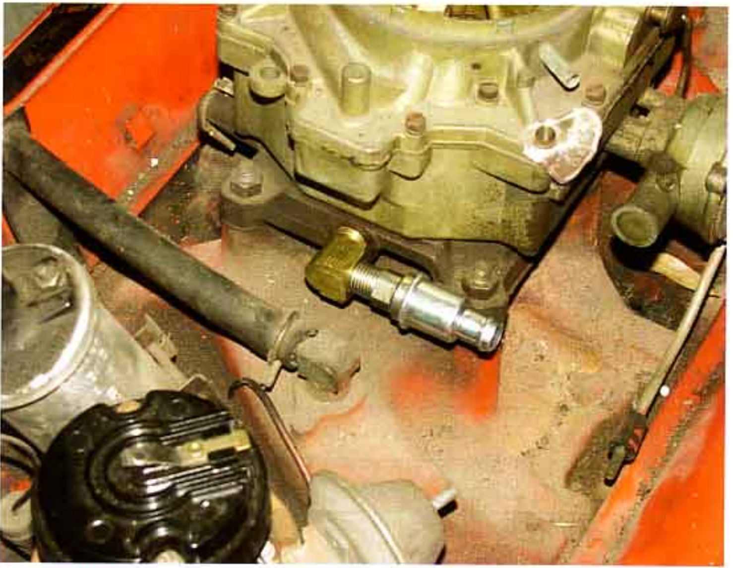
Photo #5: Install the 90-degree 1/4" pipe elbow and PCV valve supplied into the baseplate of the carburetor. Use a small amount of pipe/thread sealer on the elbow.
